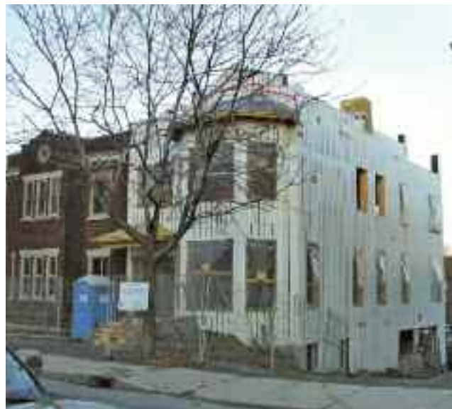
Work continues on this new semi-detached house immediately east of 536 Côte St. Antoine.
