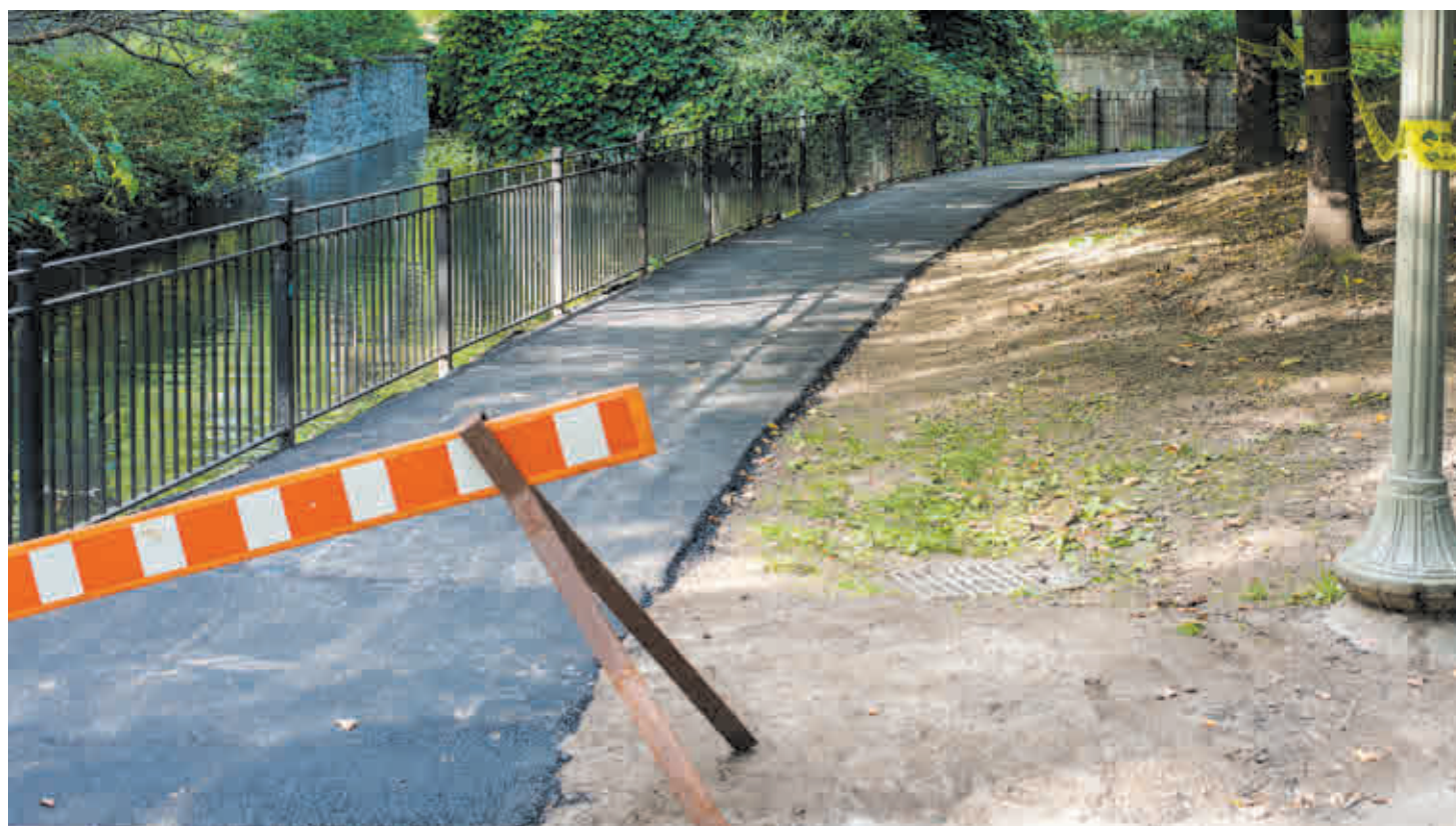
The entire length of the path on the southern edge of the Westmount Park lagoon has now been paved with asphalt, as seen here looking east from the bridge September 18.
