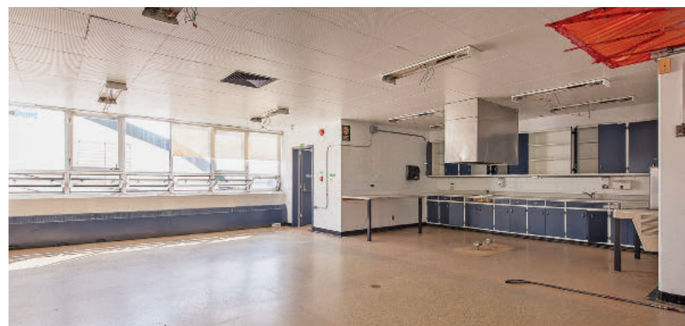
Kitchen facilities. All the equipment, chairs, tables and lighting have already been removed for the underway renovations.
