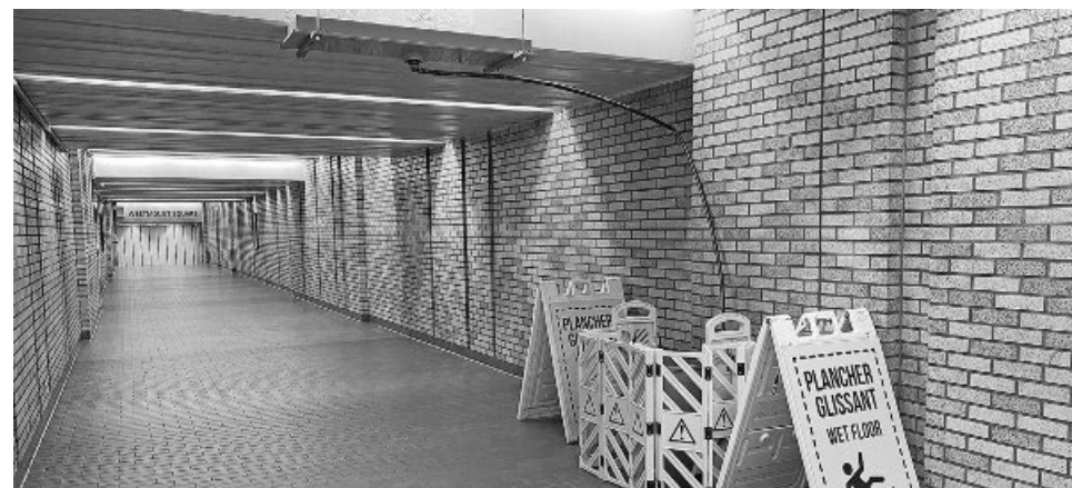
What appears to be water damage on the ceiling above a pipe that is running into a water bucket in the tunnel between Westmount Square and the Atwater Metro station, as seen August 20.
