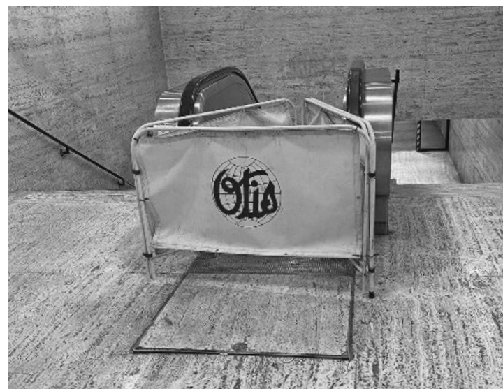
The top of the closed escalator and an "Otis" sign at the Wood Ave. entrance of Westmount Square, as seen August 22.
