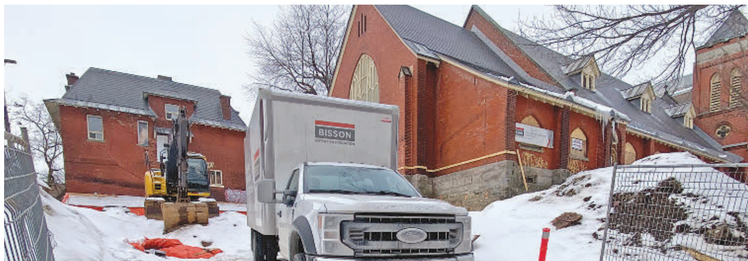
The back of the former St. Stephen's Church, right, and the site of its former church hall on March 4. The hall was demolished intentionally in 2001. The church's manse, which is a part of the development, is visible in the background at left.
