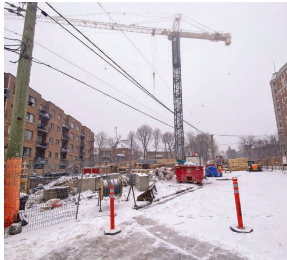
An apartment building, Le Loyal, is under construction at 4845 Côte St. Luc Rd. It is just outside of Westmount, to the northwest of the city. As seen from Bonavista Ave. looking towards Victoria Ave. and Westmount on February 27.
