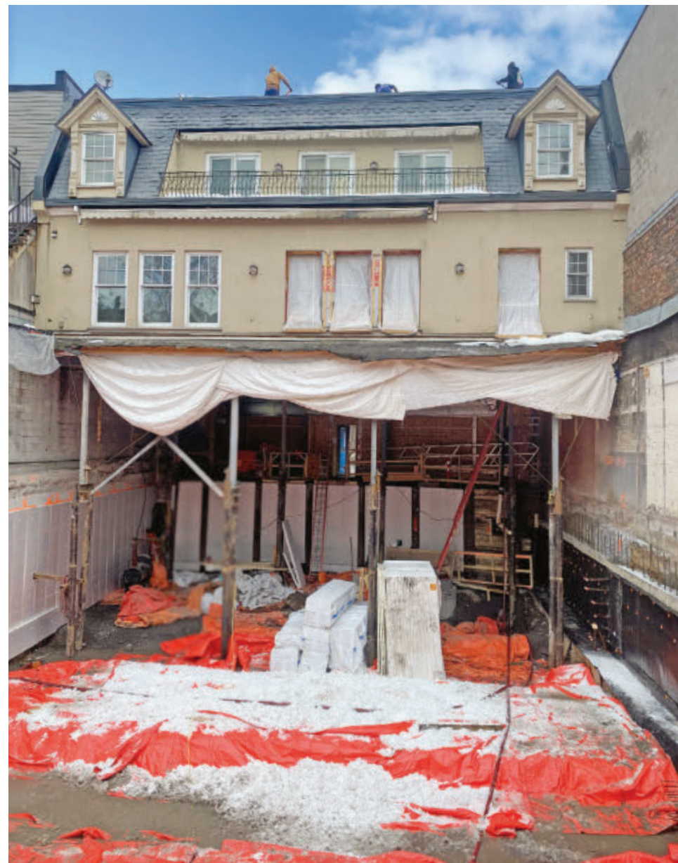
The back of 780 Atwater Ave., as seen February 26, showing an excavation of the basement and new foundation within the existing one to increase the height to accommodate rooms.
