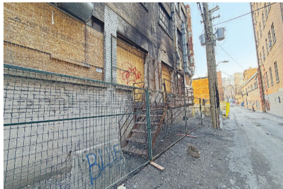
The exterior of 4024B St. Catherine viewed from the alley to the south of it showing a new fence that was erected the week of April 7, as seen April 9.
