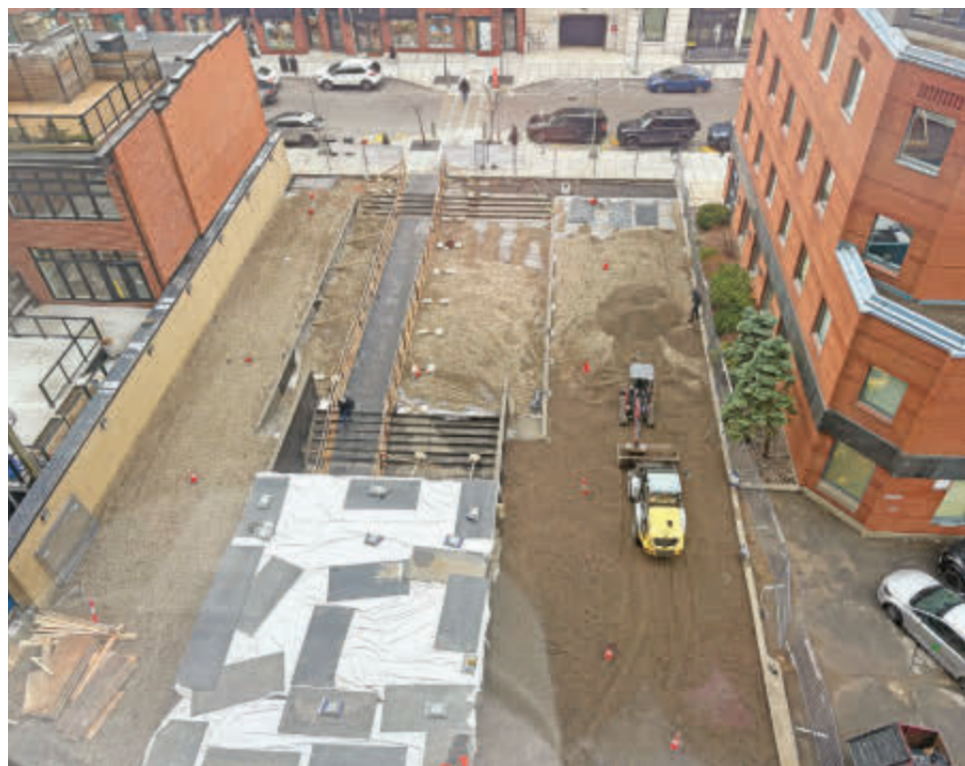
Westmount Square is the site of an $18-million infrastructure renewal program that includes a new water membrane under the exterior plaza. Work resumed on the roof of the building the week of April 13, with Greene Ave., visible at the very top of the photo (see October 21, p. SL-22, November 11, p. 10 and December 2, 2025, p. 10 for past coverage). This photo was taken April 15.
