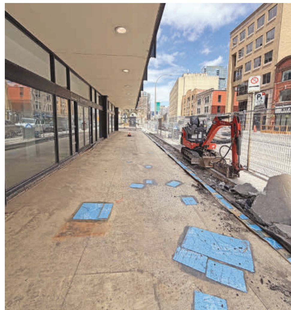
As photographed behind the chain-link fence on St. Catherine at Greene Ave., diggers are ripping up the sidewalk. As seen on May 3.
