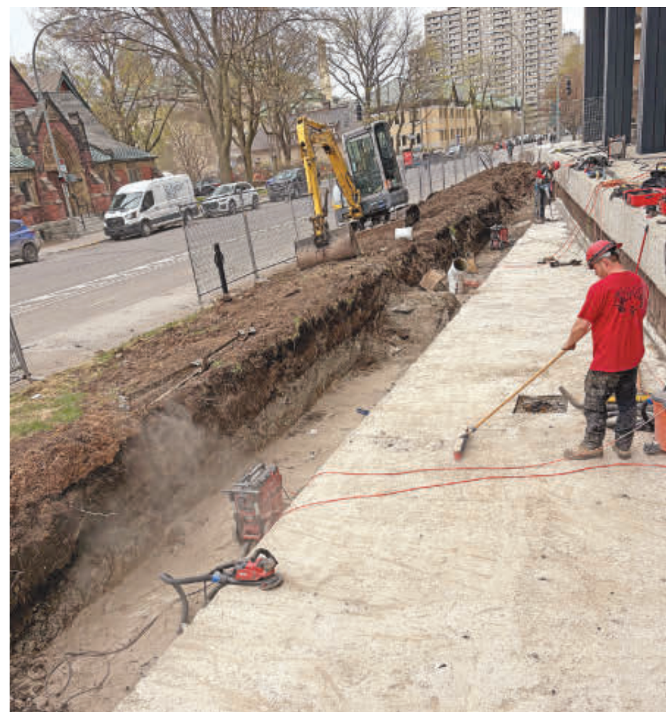
The sprinkler system has been ripped out at de Maisonneuve and Greene Ave. to be able to replace the membrane. As seen on May 3.
