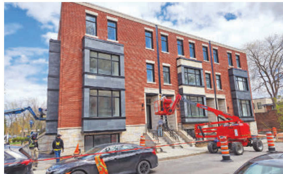
As seen May 7, work continues at Prince Albert Ave. and de Maisonneuve to complete the six-townhouse building-conversion portion of the Albert Square project, although at least one unit is occupied. The latest visible achievement is the black cladding on most of the bay windows. The two "grand" townhomes to the east, built from scratch, have been completed and one is occupied. The site's re-development story goes back to 2016 (see story June 14, 2016, p. 1).
