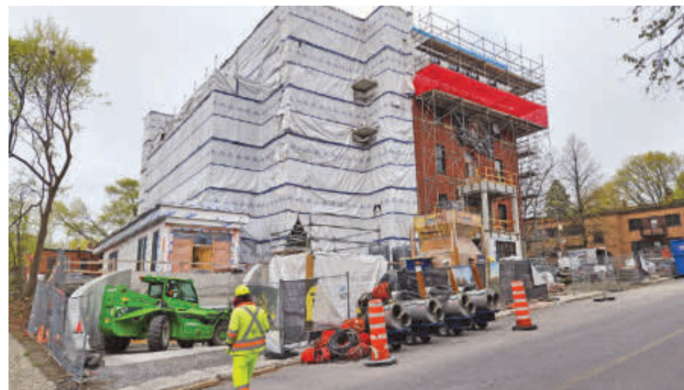
As seen May 8, work continues at the 500 Claremont residential rental project. The cross street is Windsor Ave. Its re-development story goes back to 2014 (see story February 17, 2015, p. 1).
