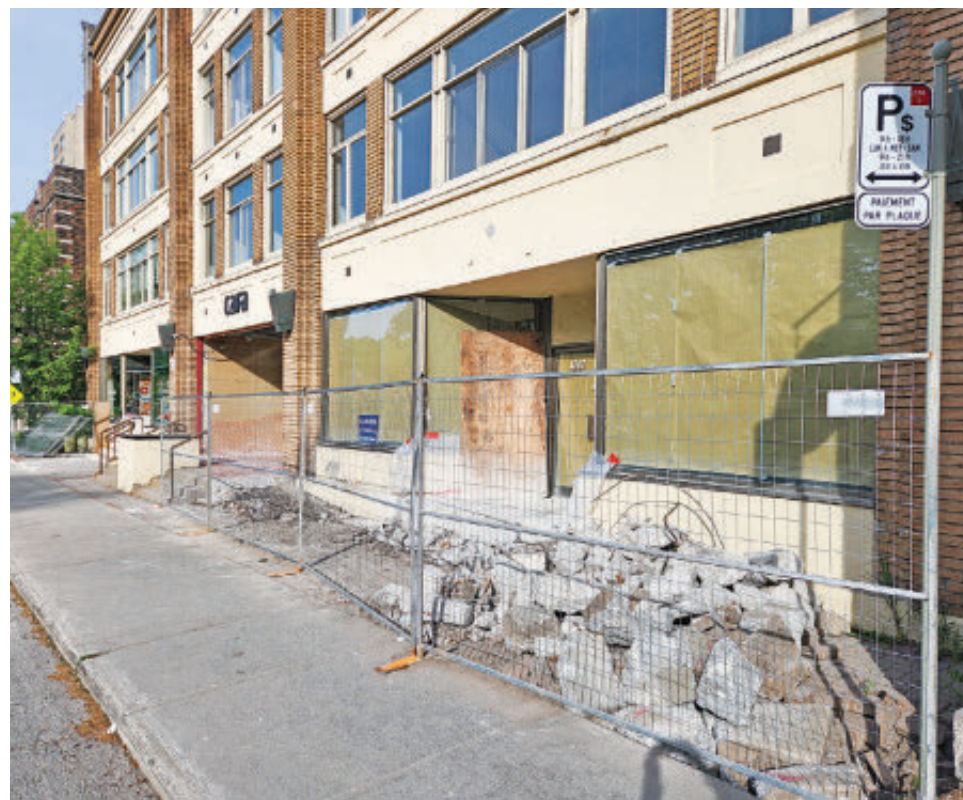
As reported recently (May 12, p. SL-23), this former St. Catherine-near-Clarke site of Atelier Fade and Save N Ship (now both on Greene) is vacant. Since our May 8 photograph, the steps have been jackhammered into oblivion, as seen May 23, presumably to facilitate some sort of renovation.
