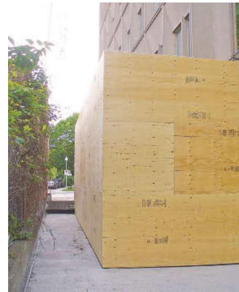
The new structure at 245 Victoria encasing its ventilation equipment on June 5. This view is from the parking lot behind the building, but it is also visible from the street.
